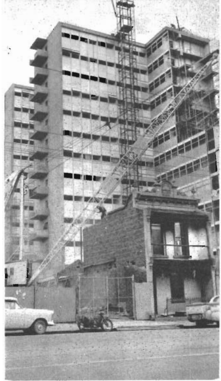
The old and the new : Demolition of old buildings in Carlton to make way for the new wing of the Royal Women's Hospital.
